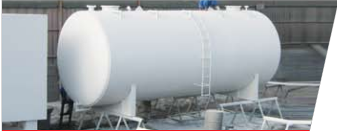
ACID STORAGE TANK
